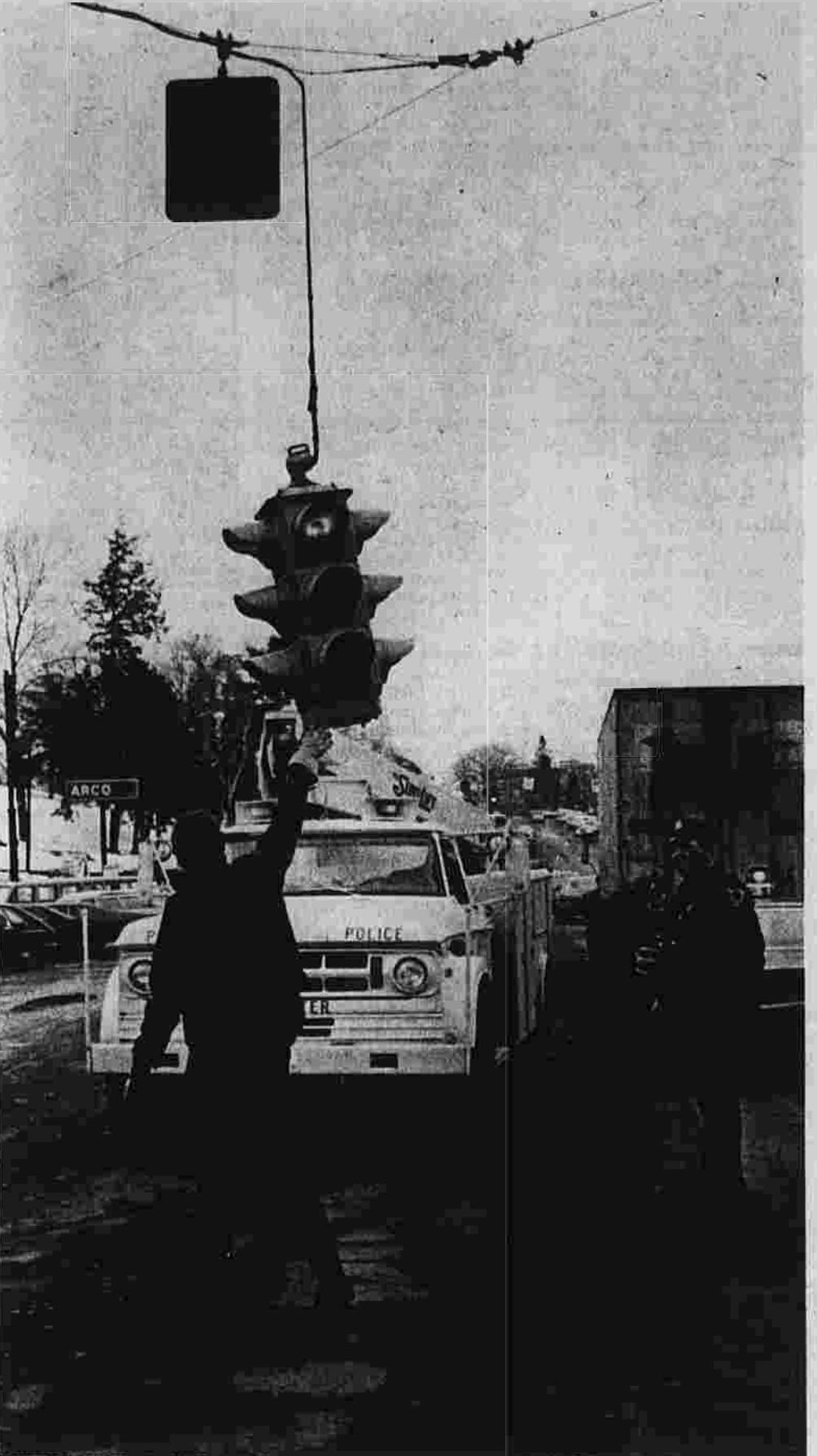
The Truck Was Too High
